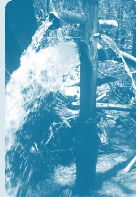
Image 1. Water running out of an uncapped bore
